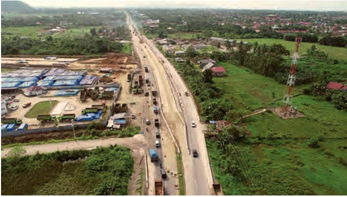
▲ Aerial photo of the Trans-Sumatra toll road under construction. (Image courtesy: Hutama Karya)
