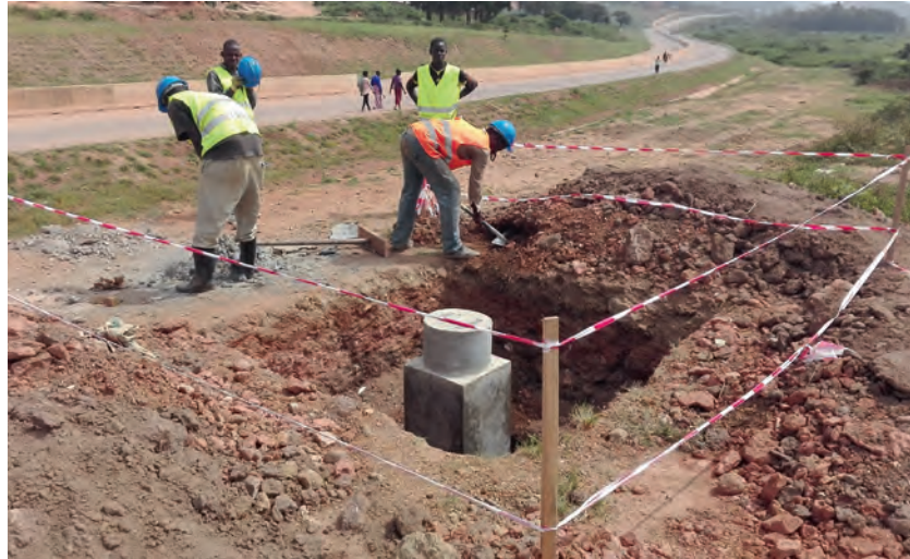
▲ Figure 3: Construction teams set up geodetic monuments in accordance with HSSE best practices.
